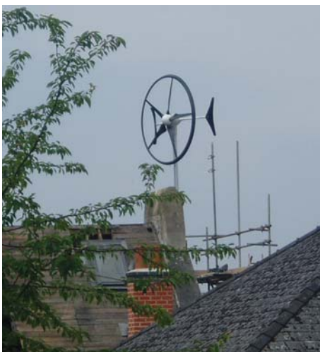
Domestic wind turbine
